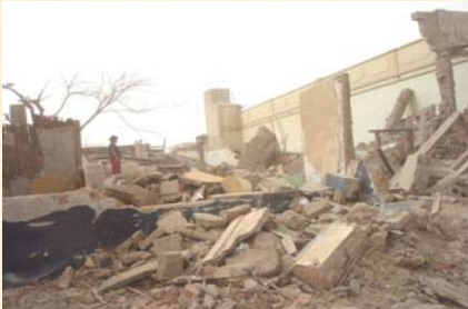
Collapsed adobe houses in Pisco
