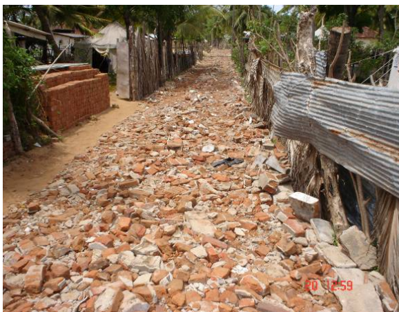
Photo 1: Dumping of unprocessed tsunami debris for road construction – a wasteful process.
